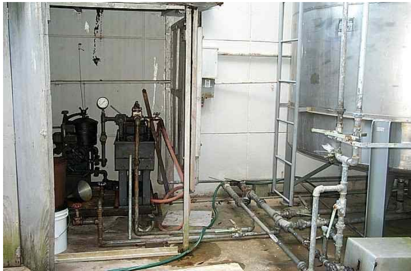
Oil purifier/filter in shelter next to one of the two stainless steel oil storage tanks.
