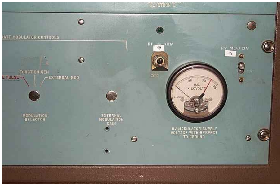
Modulator disable: small slide switch at the right of the modulator high voltage supply meter
