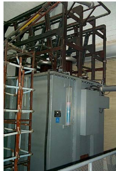
High voltage transformer (rectifiers on top)
