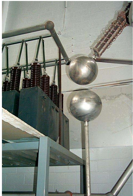
Crowbar discharge balls. Capacitors at left are part of the capacitor bank.
