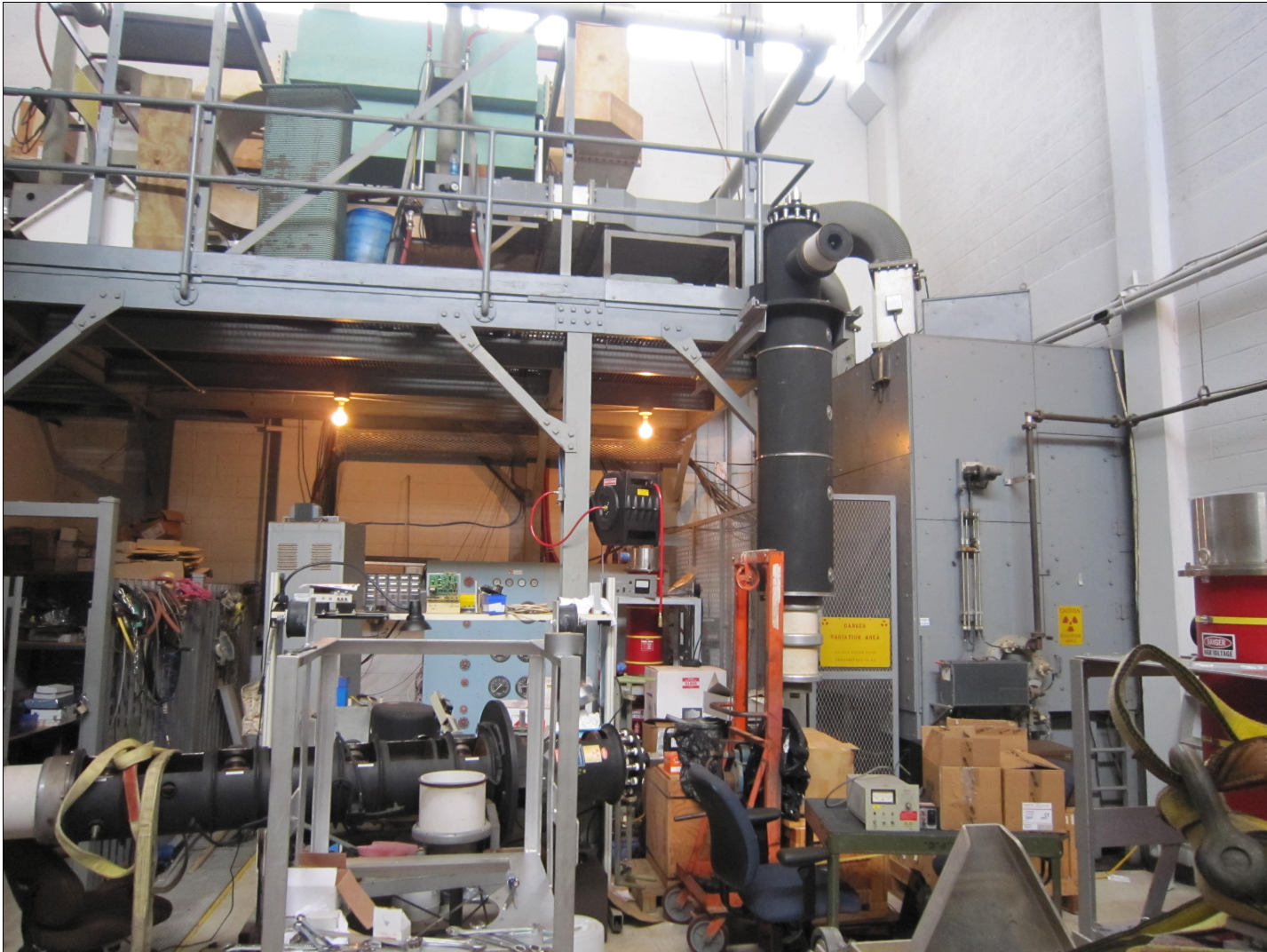
Figure 4 The 430 MHz Klystron cabinet with yellow caution radiation signs.
