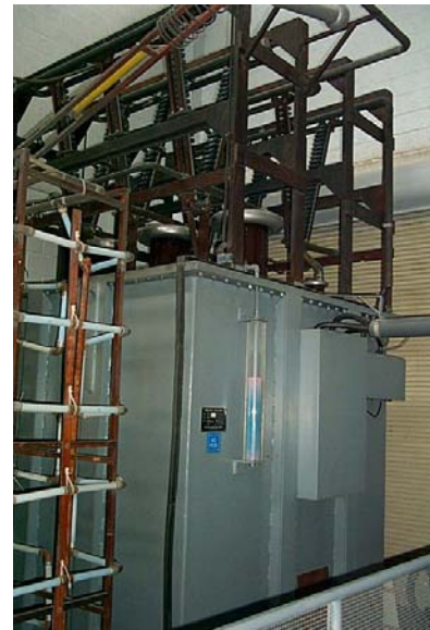
High voltage transformer (rectifiers on top)
