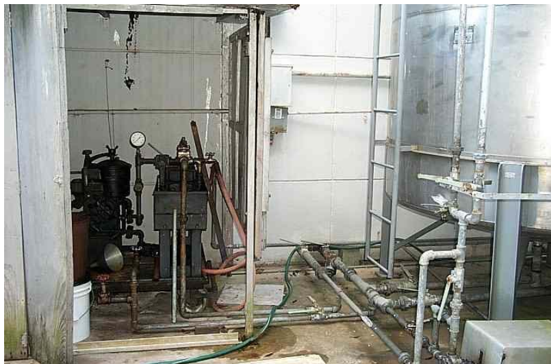
Oil purifier/filter in shelter next to one of the two stainless steel oil storage tanks.
