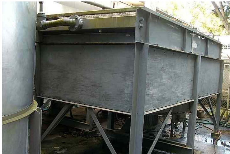
Heat exchanger on pad next to oil storage tanks.
