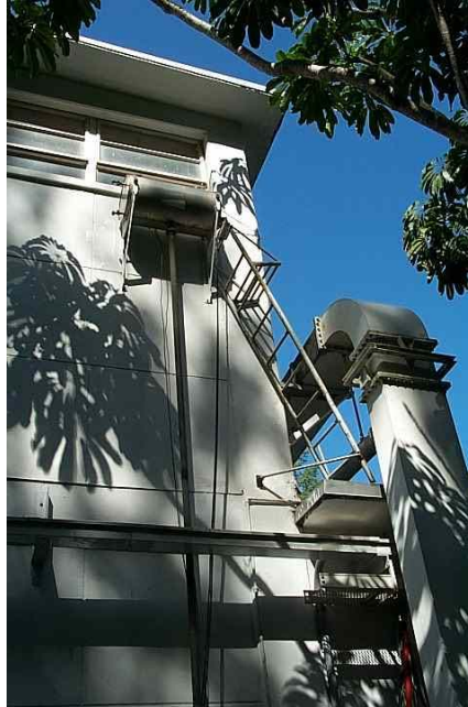
Water storage tank on side of building. Note the waveguide, leaving the EH tuner on the mezzanine and heading down to loop beneath the road.
