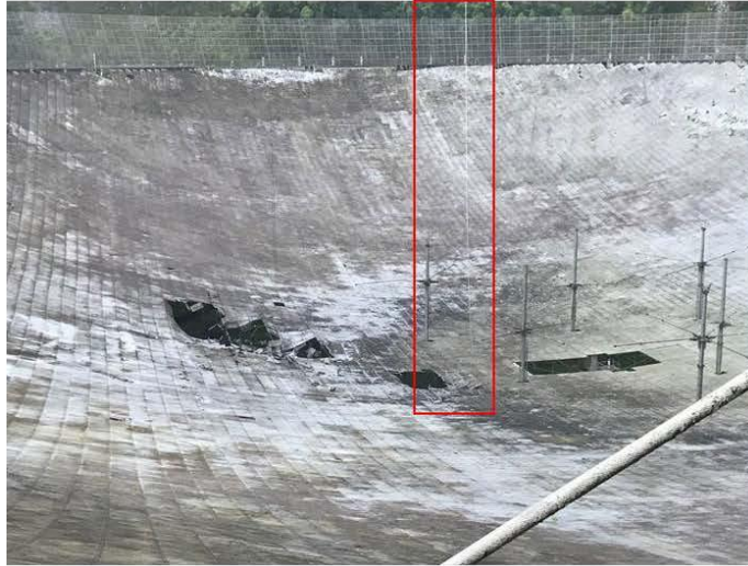
Figure 9. Photo of the failed M4N auxiliary cable, where the Tower T4 connection came to rest on the observatory dish below the Feed Platform. This photo was taken prior to the ultimate collapse of the observatory. Photo provided by WJE.
