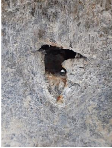
Figure 7.2.5-5 (Appendix A Figure 100). Corrosion around Wire Hole
