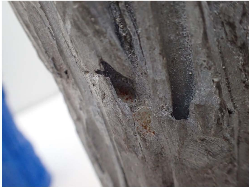
Figure 154. Close up view of a couple wire fractures on the 12 o'clock side of the cable-end section.
