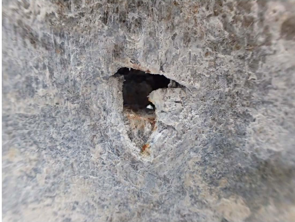
Figure 100. Heavy corrosion around one of the wire holes that breached the zinc casting outer diameter. The bright light in the center of the hole is light coming from the center of the socket cavity.
