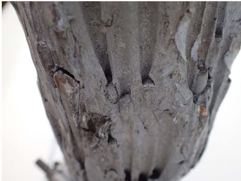
Figure 157. Close up view of wire fractures on the 3 o'clock side of the cable-end section.
