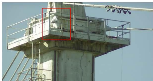
Figure 7. Photo, provided by WJE, of the failed M4N socket, prior to removal from Tower T4. The socket was retrieved prior to the observatory's ultimate collapse.
