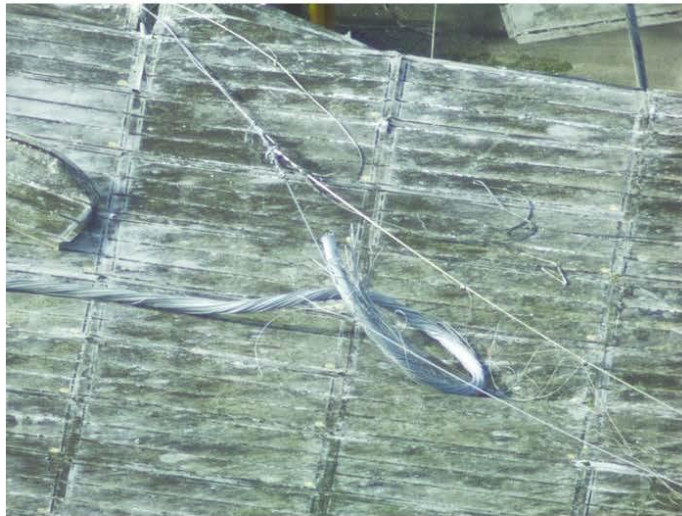
Figure 10. Close up photo of the failed M4N auxiliary cable, where the Tower T4 connection came to rest on the observatory dish below the Feed Platform. This photo was taken prior to the ultimate collapse of the observatory. Photo provided by WJE.
