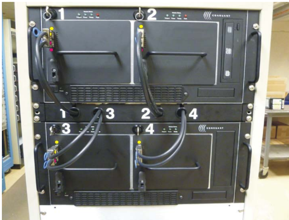
Figure 1: Front view of rack-mounted Mark 6 system (need photo including module labeling)
