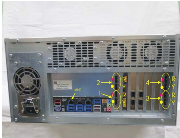
Figure 2: mini-SAS cable connections to host-bus adapter (i.e. disk interface) cards on rear of system chassis. Numbers correspond to cable tray labeling. 'R' is for red-labeled cables, 'Y' for yellow-labeled cables. Positions '3' and '4' will not be used (and may not exist) if an expansion chassis is not installed. Position of 'eth0' network connector is also shown.
